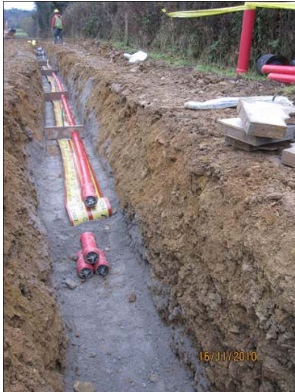
Plate 4.8 Typical Cable Trench View
