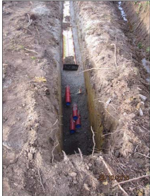
Plate 4.9 Typical Cable Trench View
